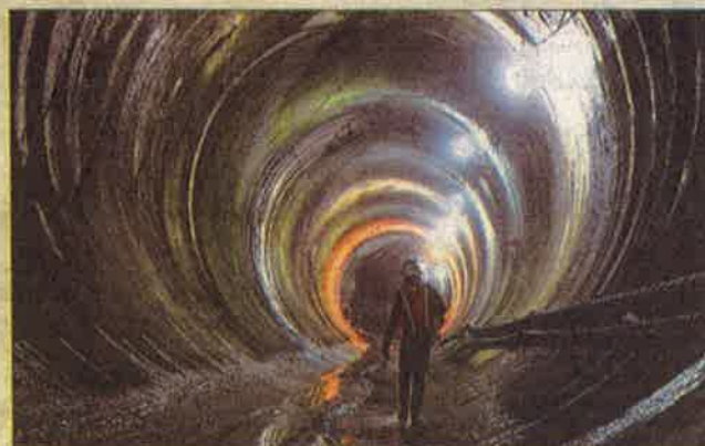
Completion of the East Side Access project linking the Long Island Rail Road to Grand Central has been delayed to 2019.
