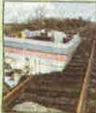
Damage on the Rockaway Line
